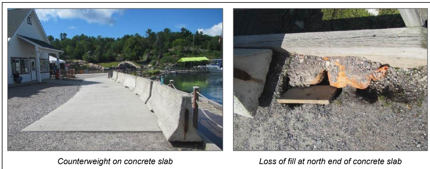
Figure 7: Example of Wharf Conditions (2020)
