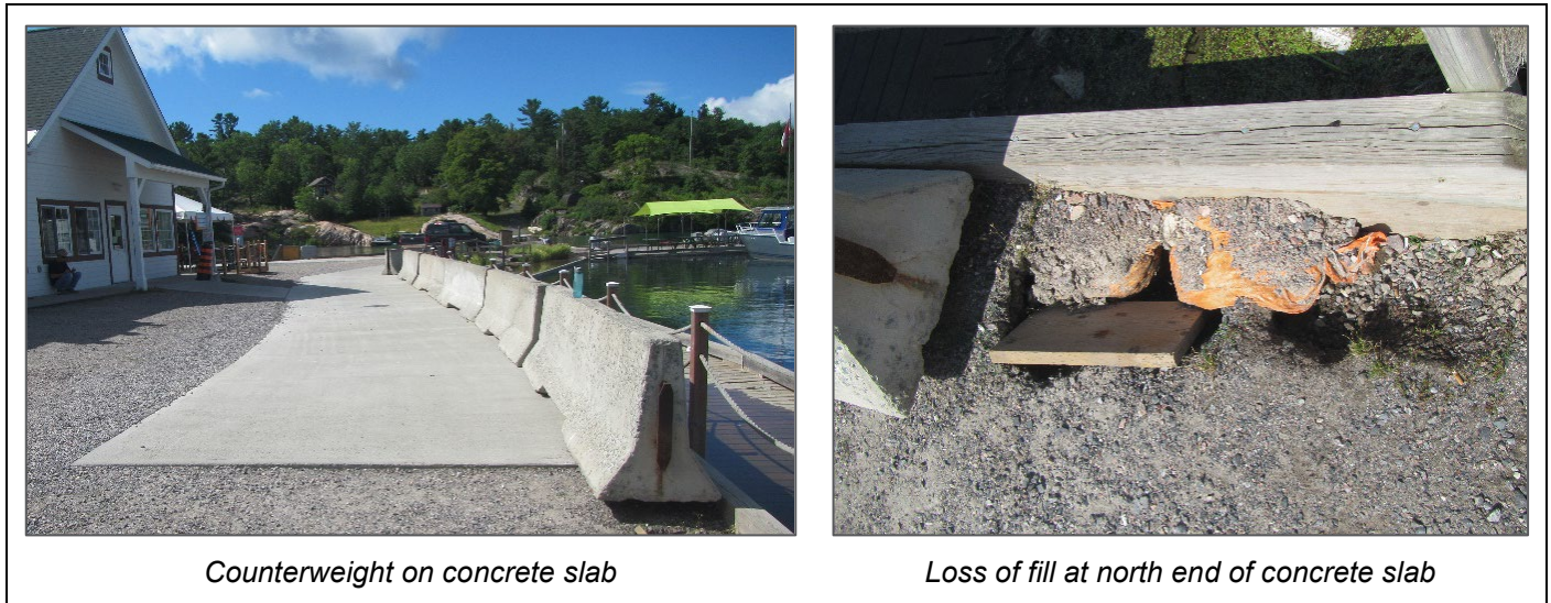
Figure 7: Example of Wharf Conditions (2020)
