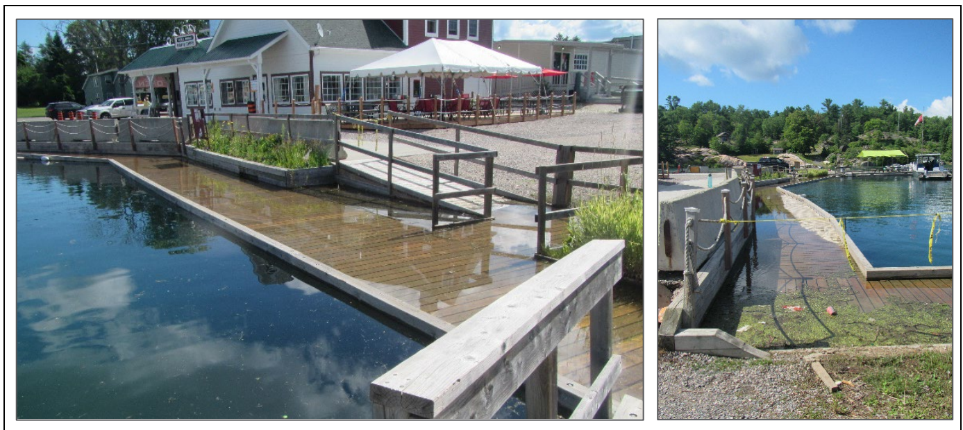
Figure 6: Flooding at the Killarney Municipal Wharf (July 2020)
