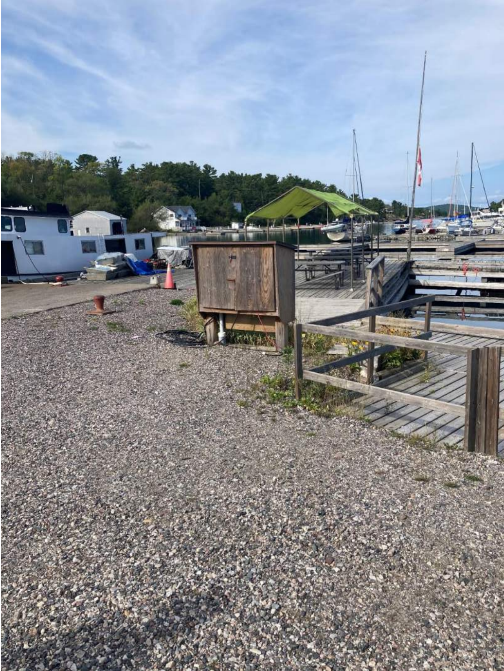
Photograph No. 9 Circuit board and electrical box in south area of Site.
