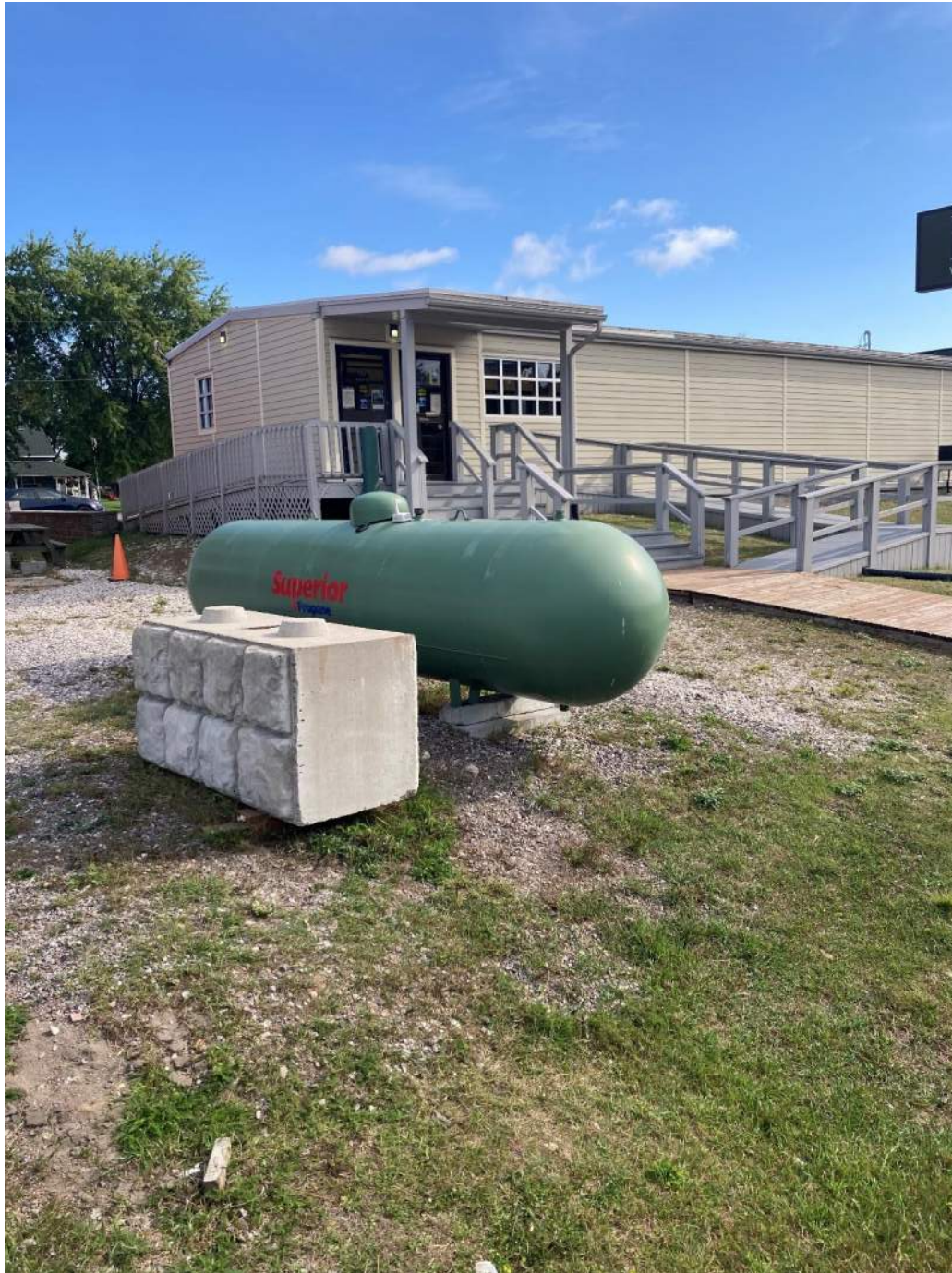
Photograph No. 6 Propane storage tank in east-central area of the Site.
