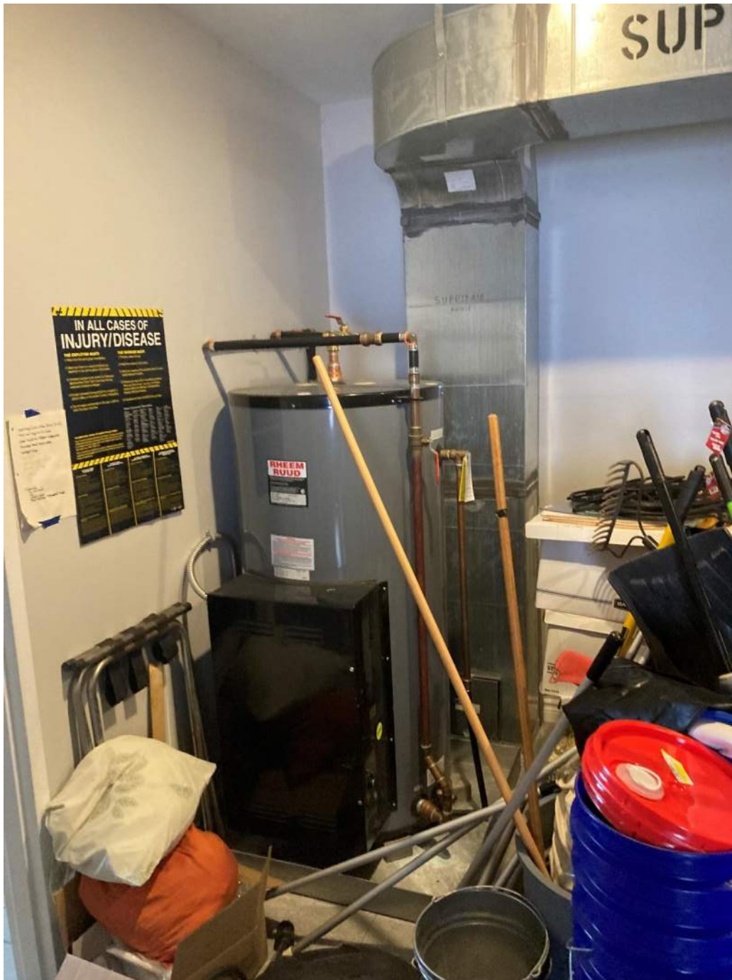
Photograph No. 14 Water heater in upstairs storage area of central building.
