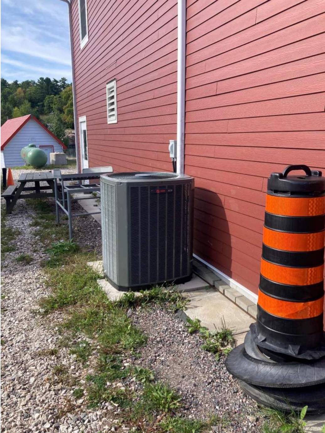
Photograph No. 11 Air conditioning unit on east wall of central building.
