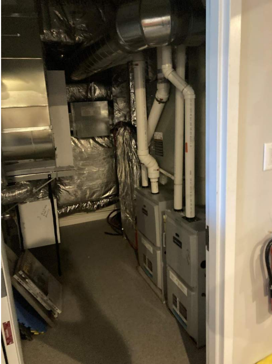
Photograph No. 13 Furnace system and controls in upstairs storage area of central building.
